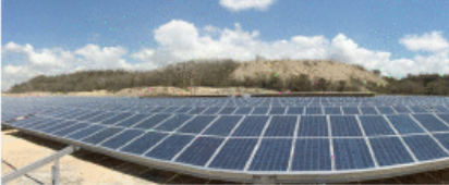
Solar energy installations. Santo Domingo Cement Plant, Dominican Republic
