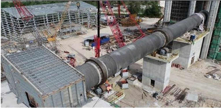
Lifting of new rotary kiln into position at Solid Cement Plant (Jan. 2021)
